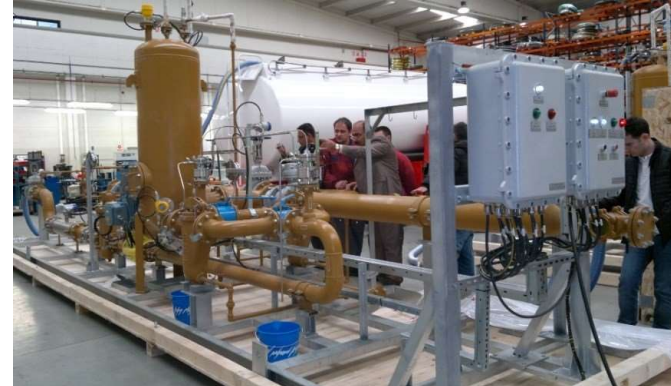
FAT for Ministry of Energy- Gasso project for power station skids
