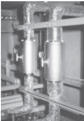
Installation in riser for lift pump
